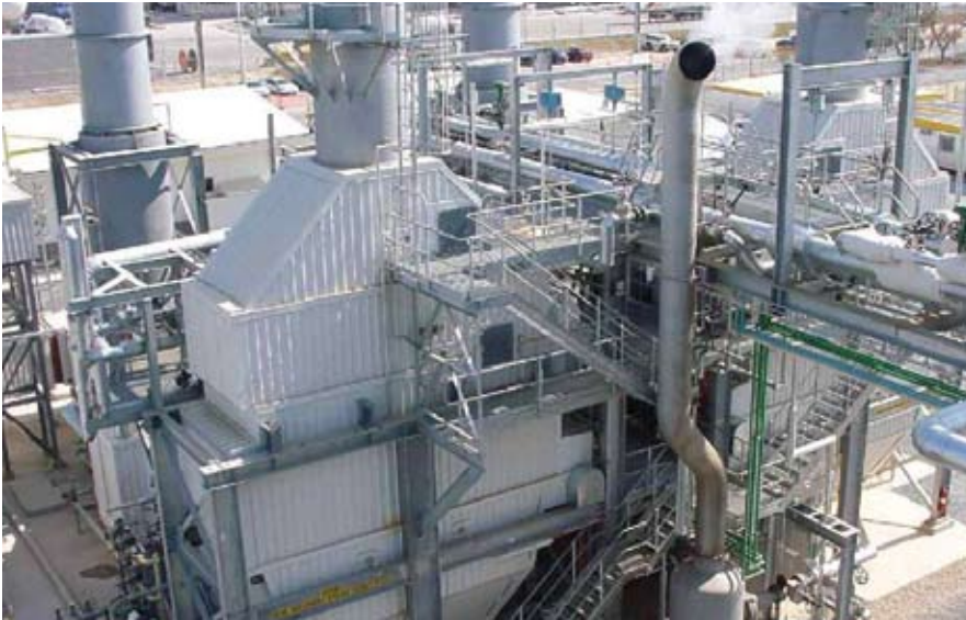
BP Refinery Bulwer Island - Brisbane, Australia
